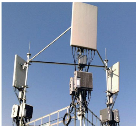
Communication base station
