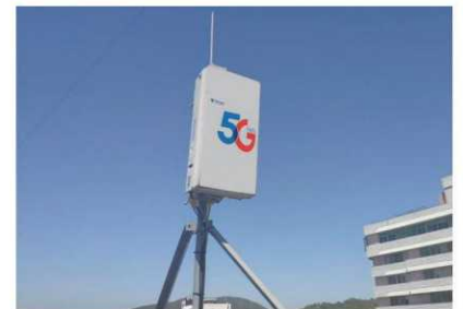
5G base station power supply
