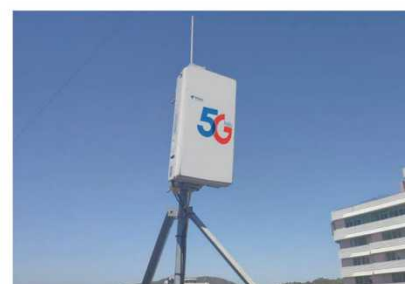
5G base station power supply
