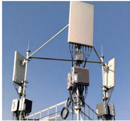
Communication base station
